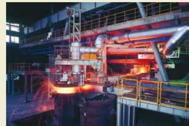
Ferronickel smelting electric furnace: The world's largest class of electric furnace, which smelts ferronickel by melting ore at a temperature of about 1,500 degrees Celsius.
