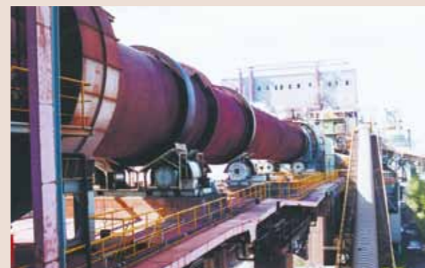
Rotary kiln: A calcining furnace machine, over 100 m in total length that thermally processes dried ore by heating it to approximately 1,000 degrees Celsius.
