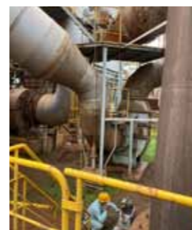
Exhaust gas measurement
