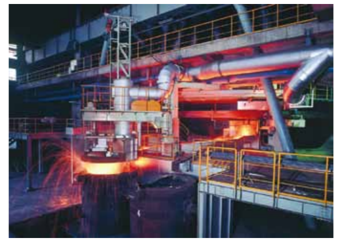
Electric furnace: These are the world's largest electric furnaces that is heated by using electric resistance, and used for smelting ferronickel from ore.
