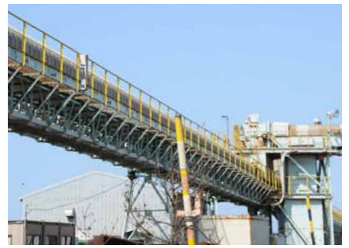
Raw material conveyor: Raw material conveyor is total around 2.4km length.
