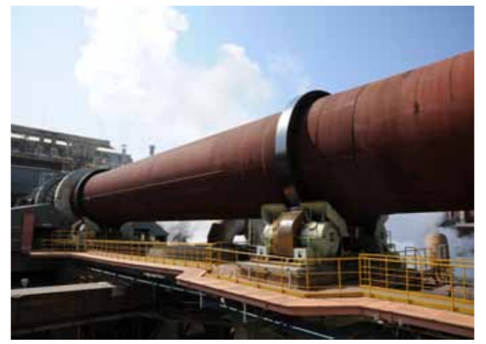
Rotary kiln: A calcining equipment, over 100m in total length that thermally processes dried ore by heating it to approximately 1,000 degrees Celsius.
