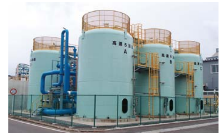
Wastewater terminal treatment facilities
