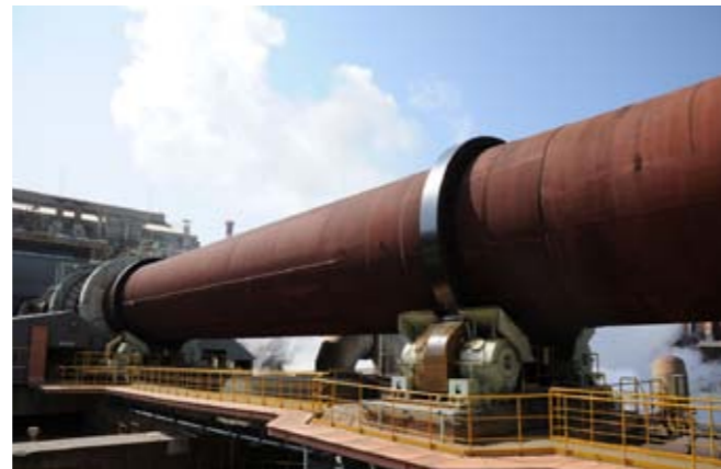
Rotary kiln: A calcining equipment, over 100m in total length that thermally processes dried ore by heating it to approximately 1,000 degrees Celsius.
