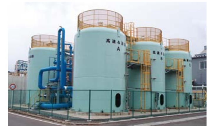
Wastewater terminal treatment facilities
