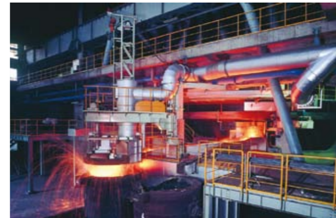
Electric furnace: These are the world's largest electric furnaces that is heated by using electric resistance, and used for smelting ferronickel from ore.
