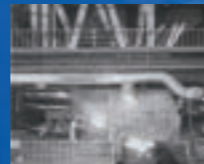
40,000 KVA closed nickel furnace (Hachinohe 45.9)
