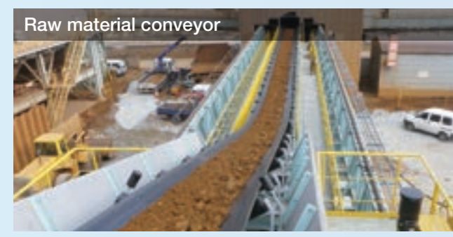
Raw material conveyor is total around 2.4km length.
