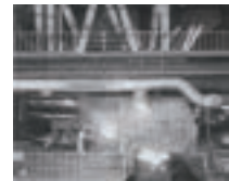
40,000 KVA closed nickel furnace (Hachinohe 45.9)
