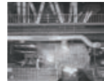
40,000 KVA closed nickel furnace (Hachinohe 45.9)
