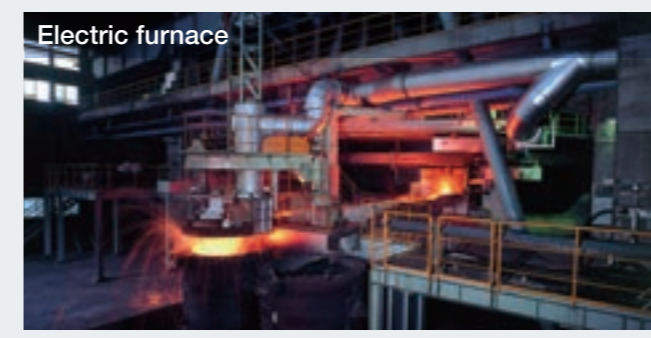
Electric furnace These are the world's largest electric furnaces that is heated by using electric resistance, and used for smelting ferronickel from ore.
